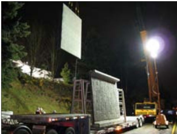
Use of extra large crane to lift panels over tree tops in order to preserve existing trees.
