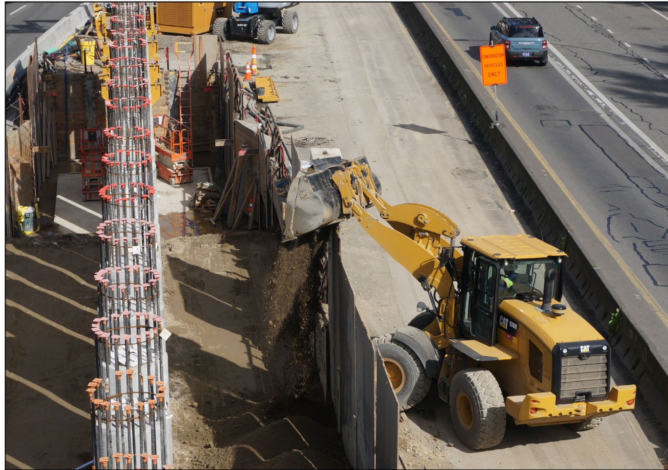
Crews work in the center of SR 520 between 10th Avenue East and Delmar Drive East to build the foundation for the new Roanoke Lid. View is looking to the east. (April 2026)
