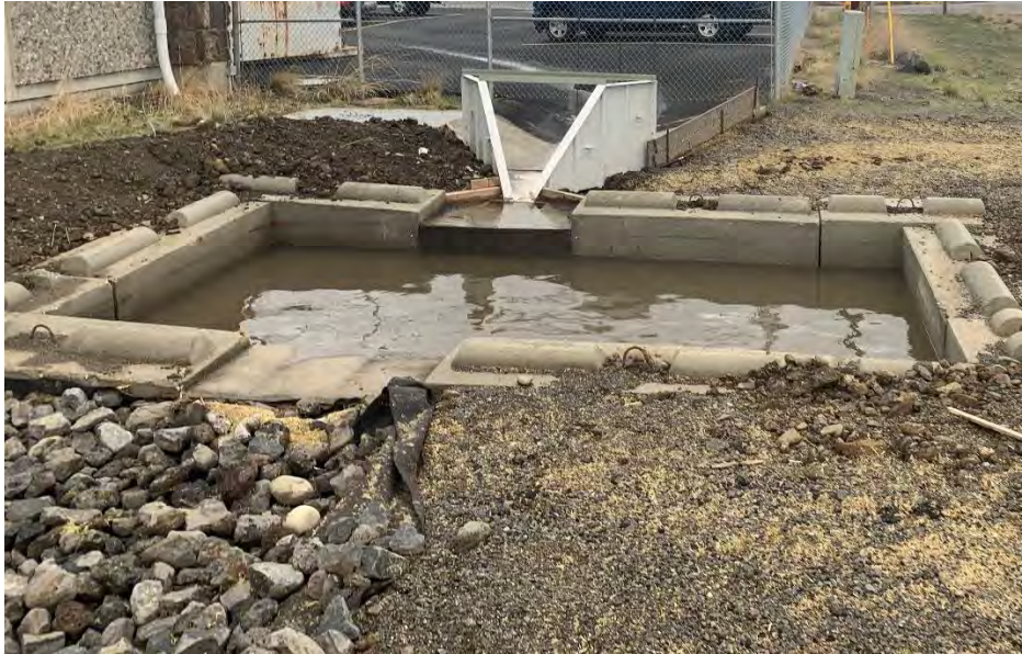
Figure 5. Geiger influent with siltation basin
