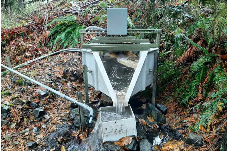
Figure 5. Mirrormont influent monitoring equipment
