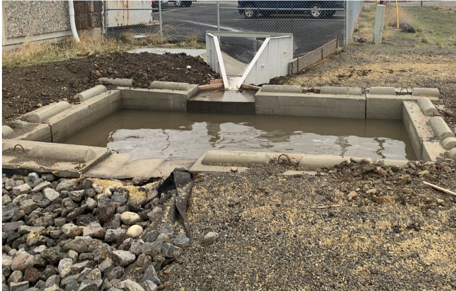
Figure 5. Geiger influent with siltation basin
