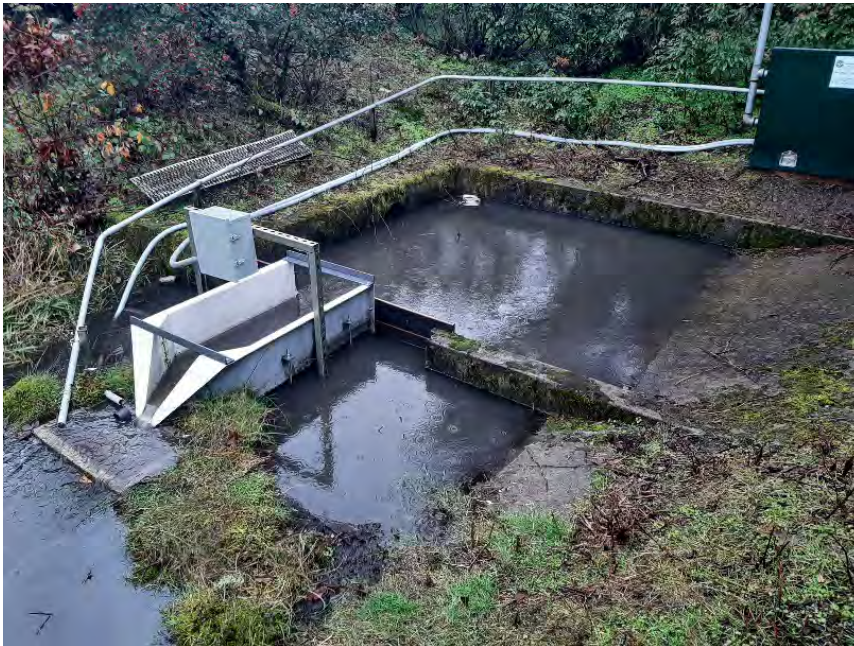
Figure 4 Vancouver influent flume and monitoring station
