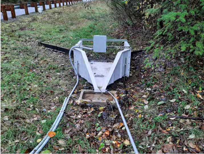
Figure 6 Mirrormont effluent flume and monitoring station
