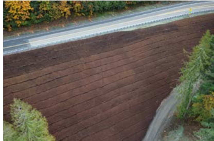
Figure 4. Slope stabilization using permeable/natural BMPs at the Elwha River Bridge project in Olympic Region.
