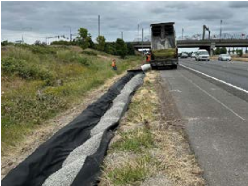
Figure 5. A media filter drain damaged by wheel path impact from heavy trucks is repaired by Southwest Region crews. Replacement of the media and vegetative strip cost $40,000.
