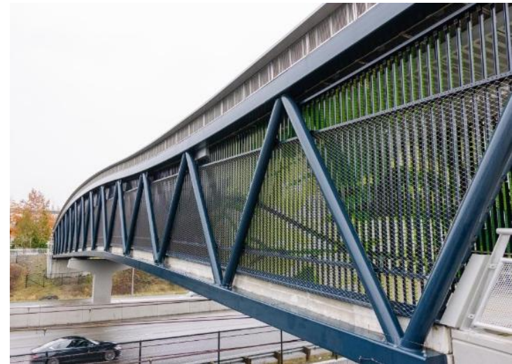
Example: Wilburton Station the Eastrail Northeast 8th Street bridge in central Bellevue will provide a critical pedestrian and bicycle crossing over Northeast 8th Street (Sound Transit)
