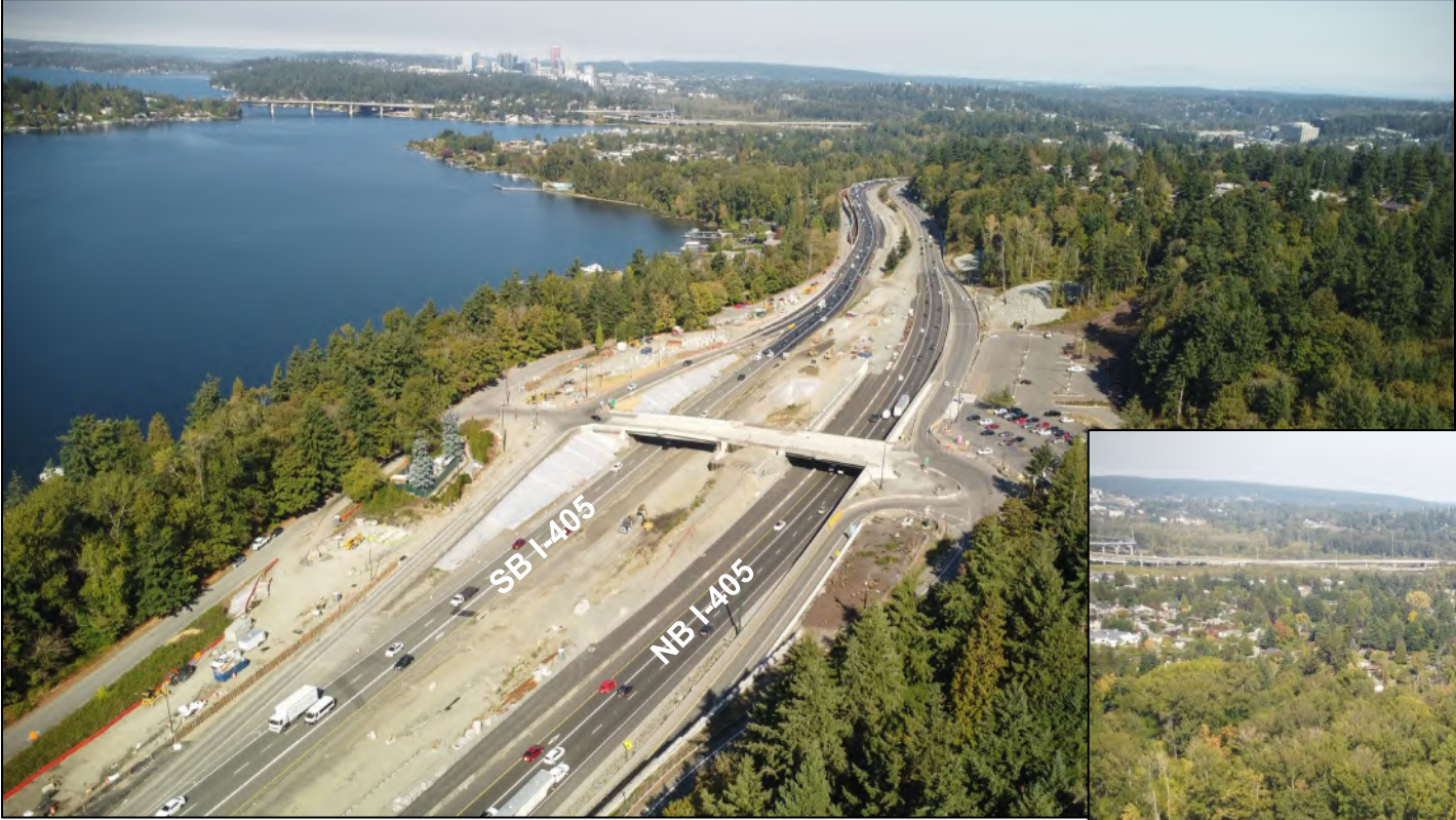
Aerial view of construction at I-405 and Lake Washington Blvd near the Newport Hills Park-and-Ride looking north
