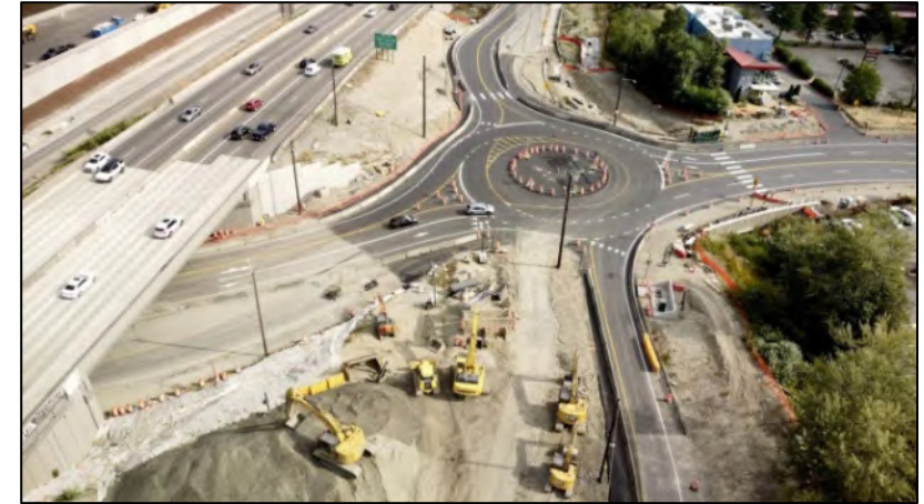
Crews installed a new roundabout at NE 44 th St and Lake Washington Blvd the weekend of July 19
