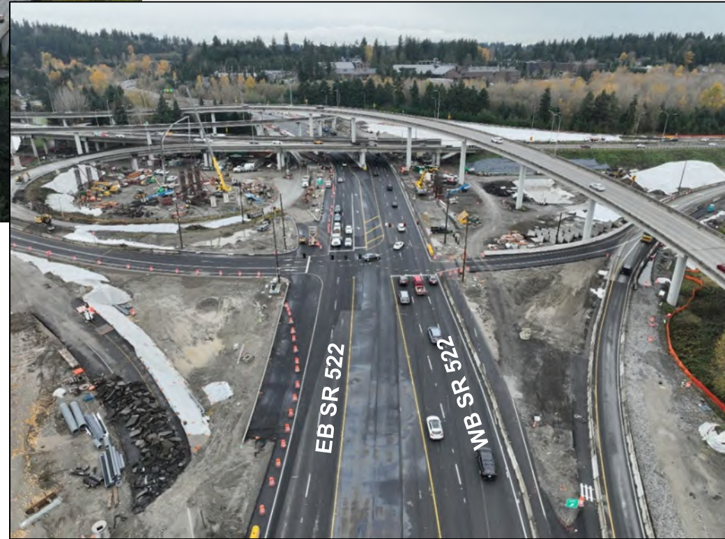
View of new traffic signals on SR 522 looking west
