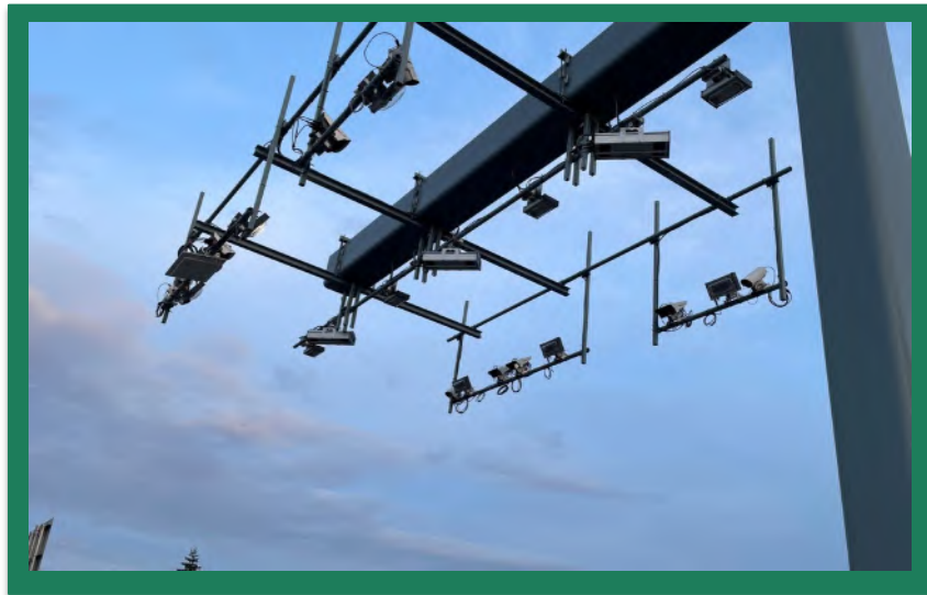
Toll gantry showing updated tolling equipment
