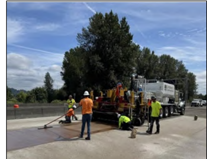
Crews replaced bridge joints and resurfaced the Green River Bridge the weekend of July 25
