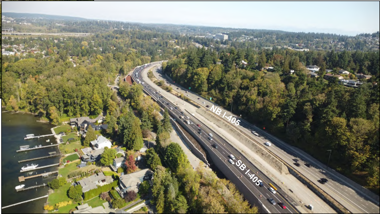
Aerial view of I-405 looking north showing work transitioning to the median
