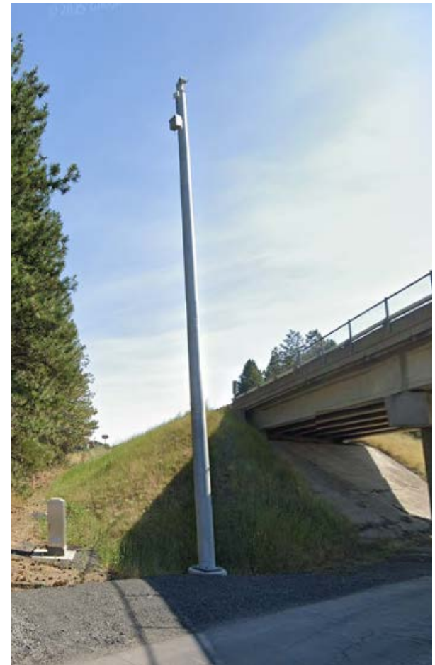
CCTV installation on pole at SR 904 and White Rd
