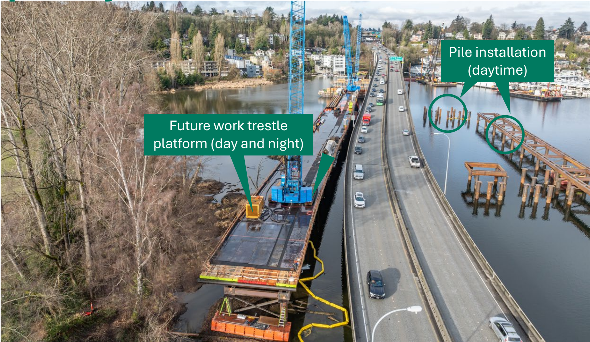
Crews have installed piles in Portage Bay to support the temporary work trestle.
