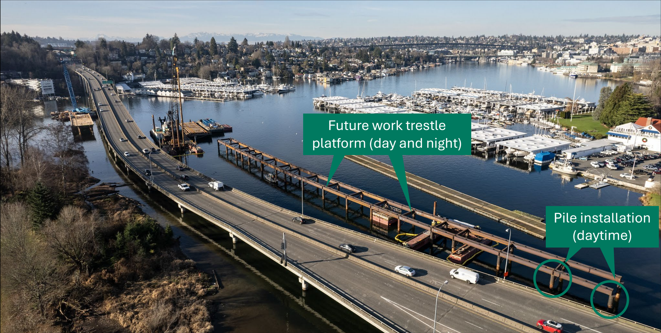
Crews have installed piles in Portage Bay to support the temporary work trestle.
