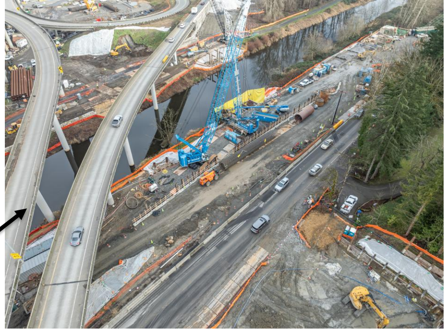
Looking east, crews work on the south side of the Sammamish River, next to Woodinville Drive.
