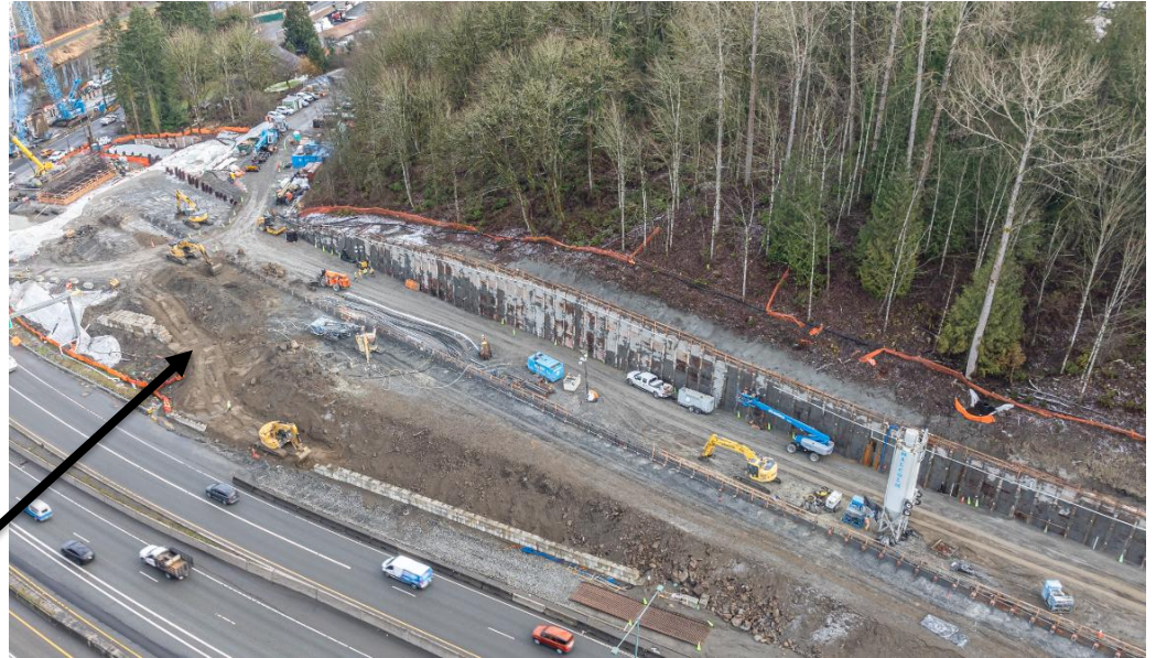
Looking northeast at soldier pile and tieback wall construction along northbound I-405.
