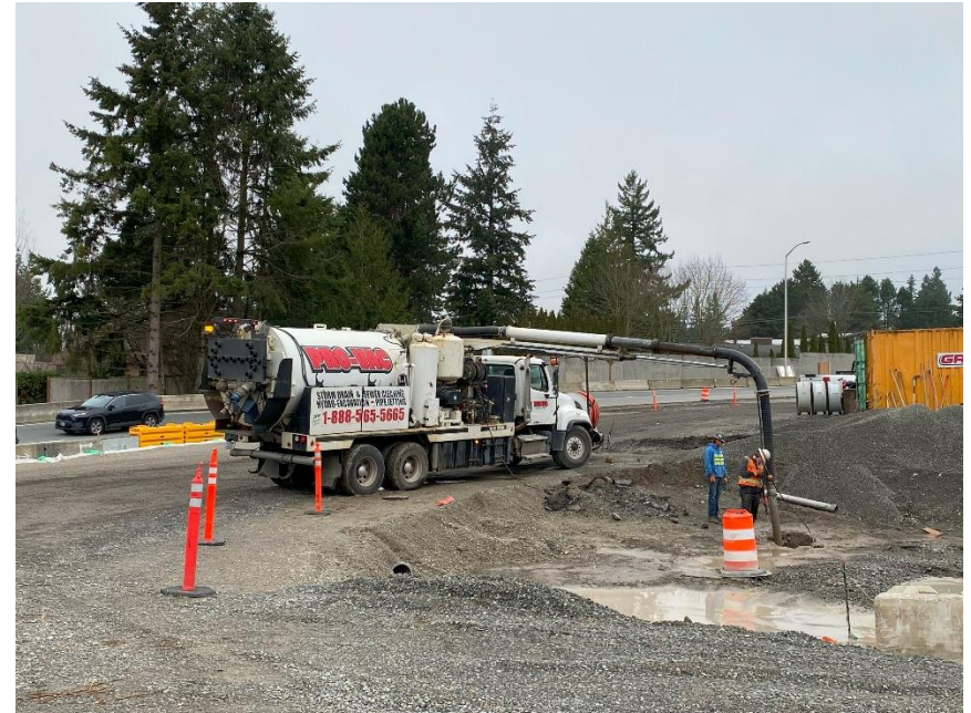
Vector truck crew working near the southbound I-405 off-ramp to Northeast 85th Street.
