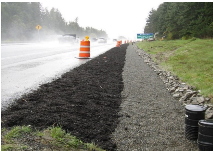
Media filter drain
