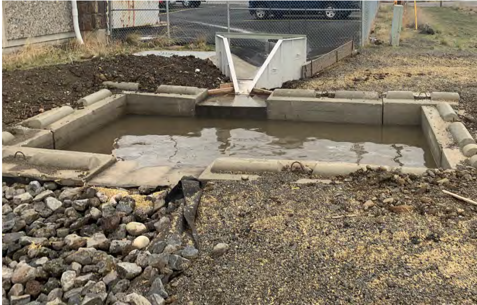
Figure 5. Geiger influent with siltation basin
