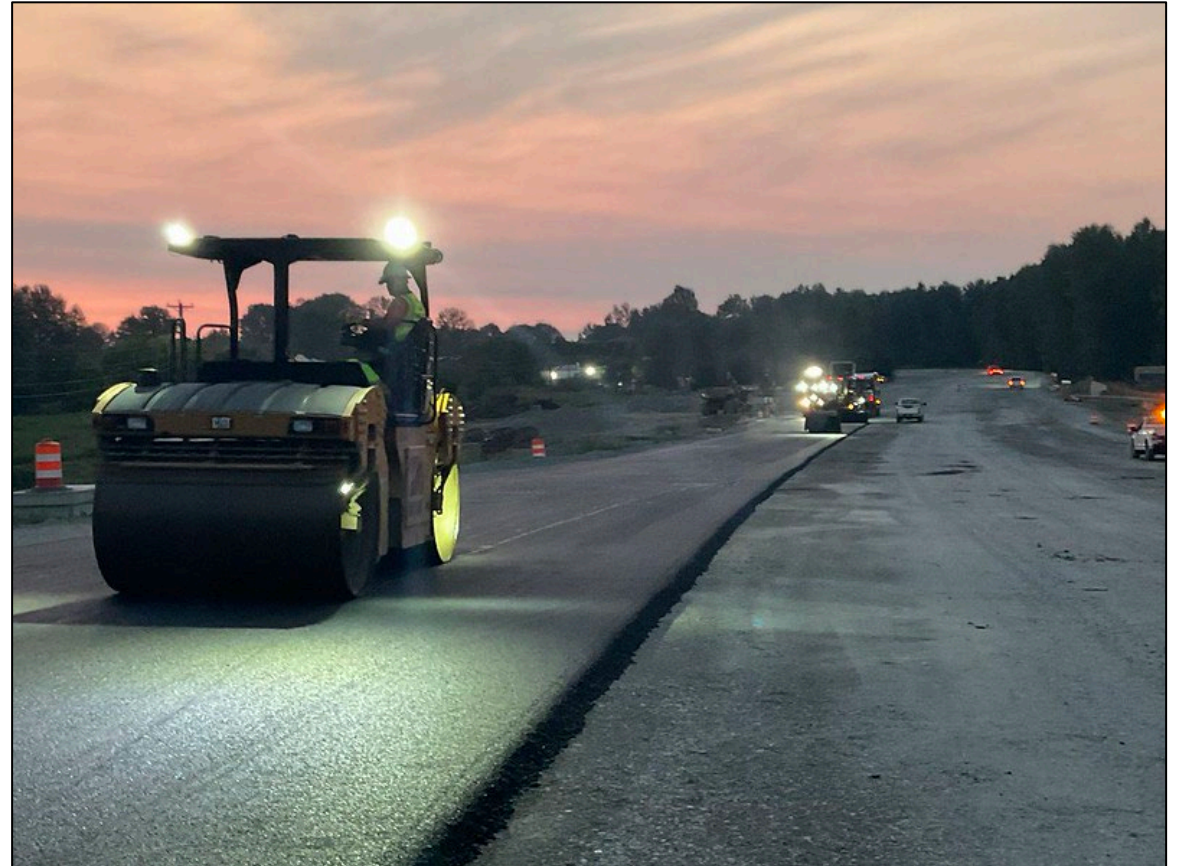
A roller is used in the early morning to help pave a new expressway in Pierce County.
