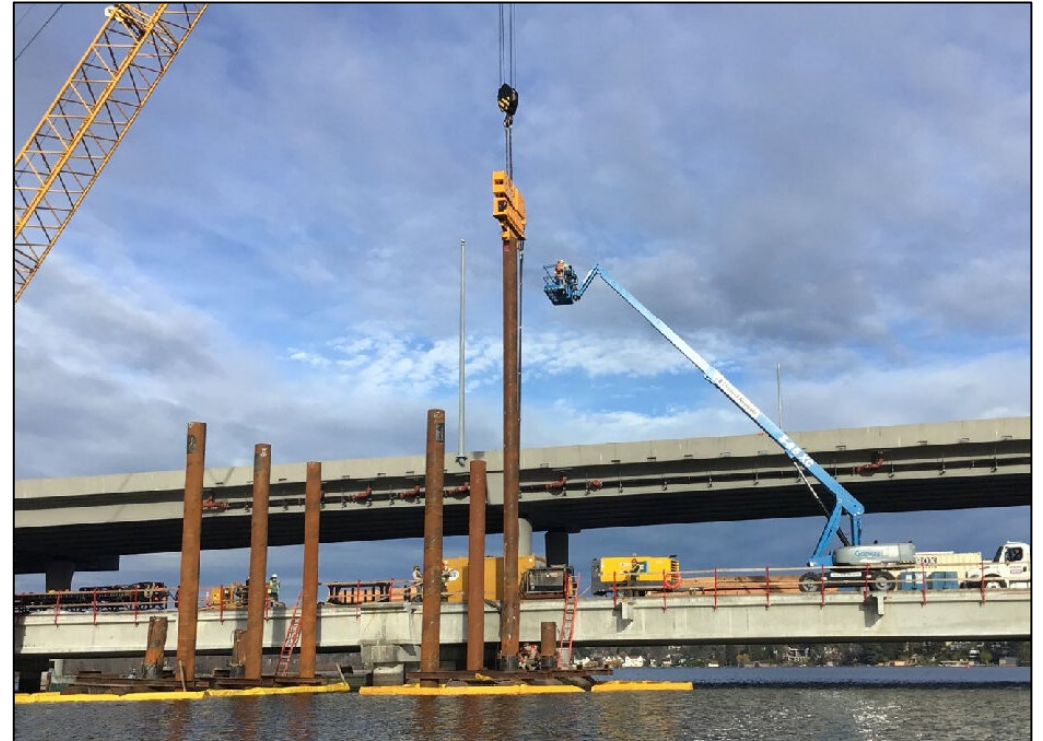
Crews use a vibratory hammer to build a work trestle during work on the SR 520 Bridge over Union Bay.
