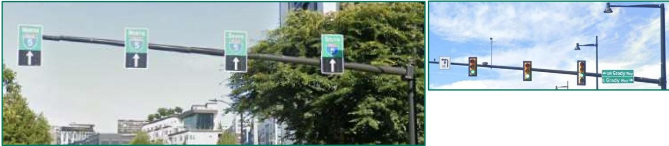
Signal mast arm: Horizontal arm bolted to vertical pole that supports traffic signals, signage, or other equipment used over traffic at intersections and along roadways. Pictured above (left to right): Signal mast arm with signs only on Mercer St. in Seattle; signal mast arm supporting signals and signs on Grady Way in Seattle.
