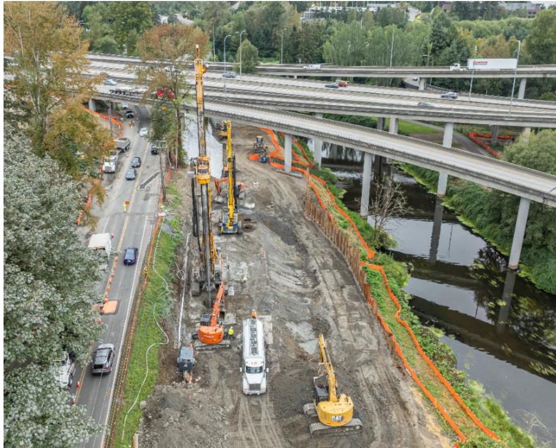
Looking west, crews work on the south side of the Sammamish River, next to Woodinville Drive
