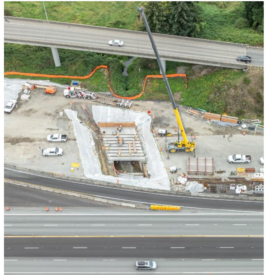
Looking north, a section of the new Par Creek Fish Passage under SR 522
