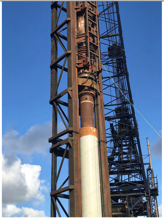
Plate 2 – Impacting Reinhall pile P-02N using Delmag D62-22 impact hammer on 2/8/2021. Note 18" O.D. mandrel inside the structural pile was directly impacted by the diesel hammer.
