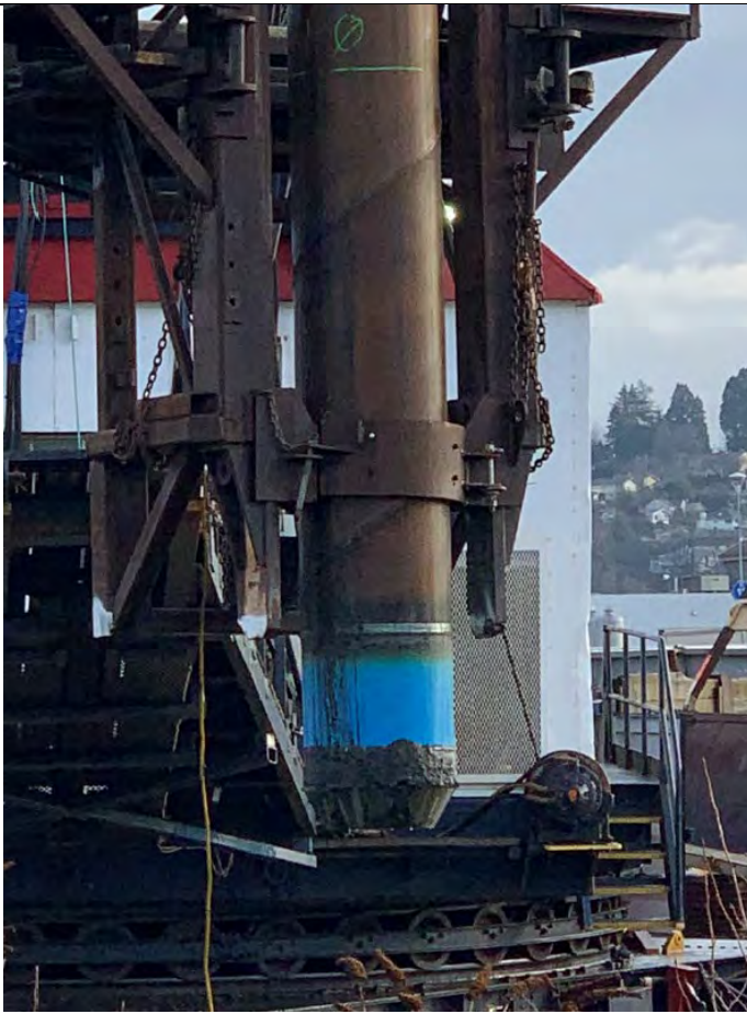
Plate 1 – Impacting Reinhall pile P-02N using Delmag D62-22 impact hammer on 2/8/2021. Note about the bottom of the structural pile attached to a 3-foot-long tip assembly with inner rings. The inner rings of the structural pile were impacted by the (inside) mandrel during pile driving.
