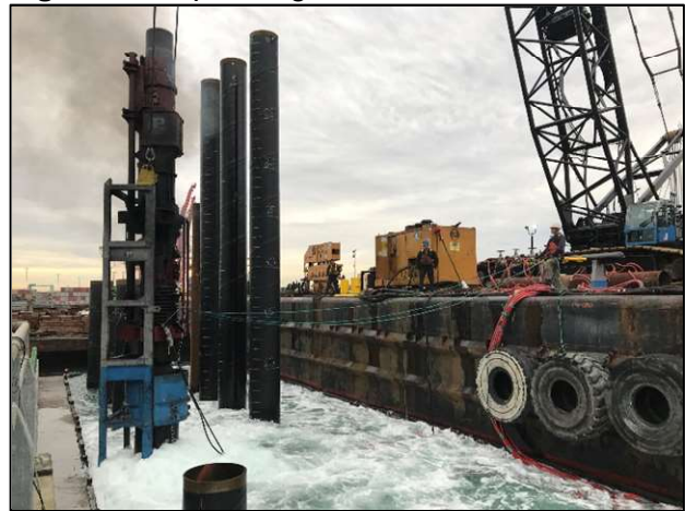
Figure 5.2 Operating Bubble Curtain
