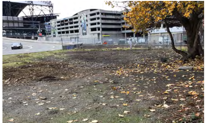
(After image): Interstate 90 near milepost 2 in Seattle. This work was coordinated by WSDOT maintenance staff and performed by a contractor on Dec. 9, 2022.
