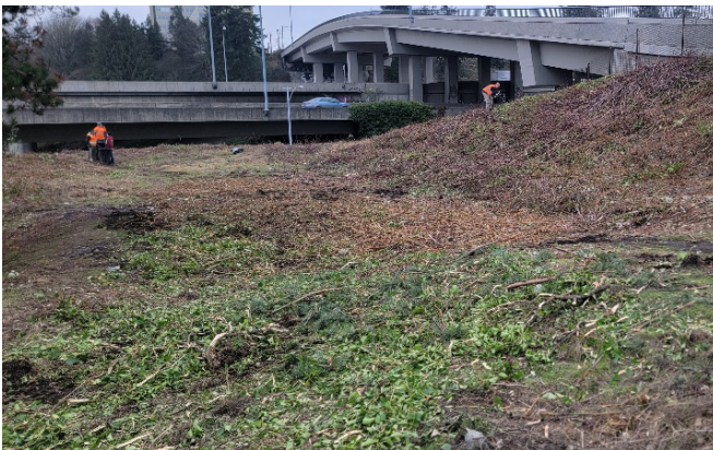
(After image): Under the SR 705 and I-5 interchange in Tacoma. This work was coordinated by WSDOT maintenance staff and performed by a contractor on Jan. 23, 2023.
