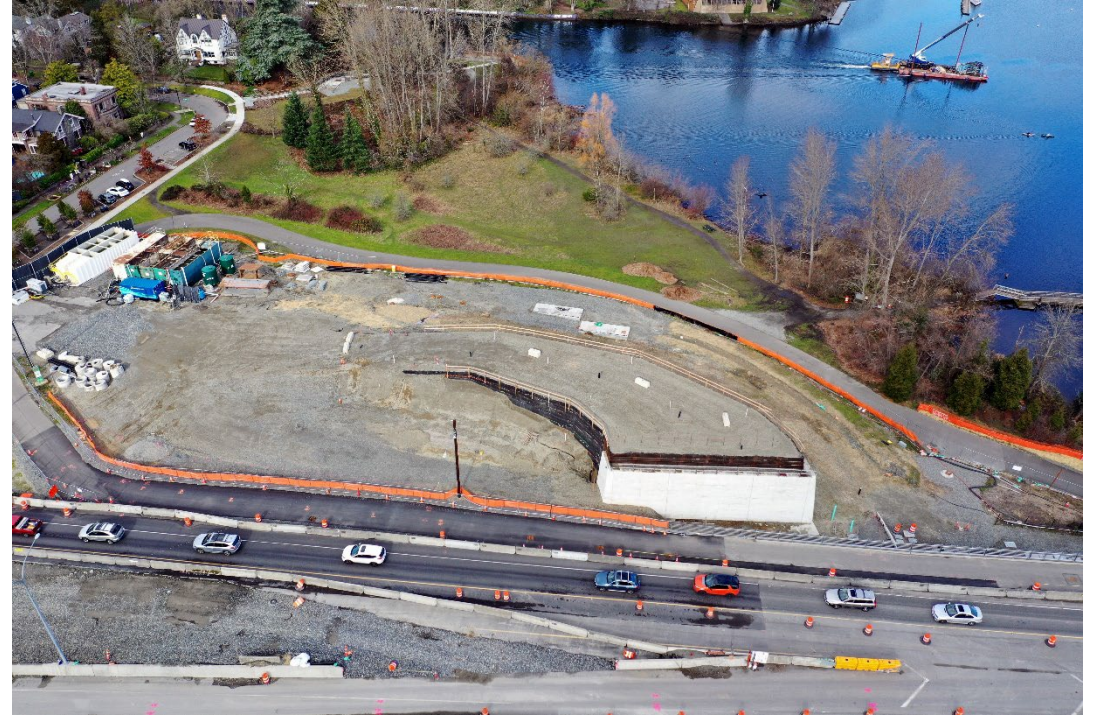
The bicycle and pedestrian bridge is starting to take shape in East Montlake Park.
