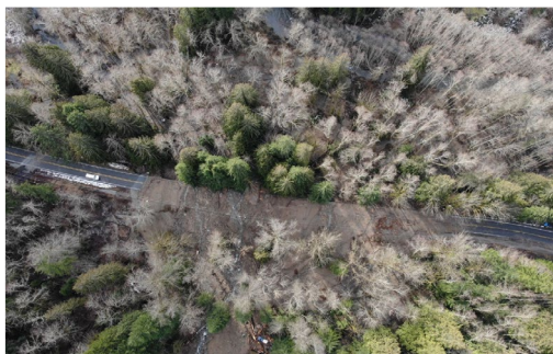
2020 Western Washington Winner SR706 / E of Ashford – Stabilize Slope
