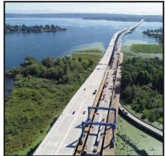
Aerial view of SR 520 eastbound bridge construction over Foster Island, looking east.
