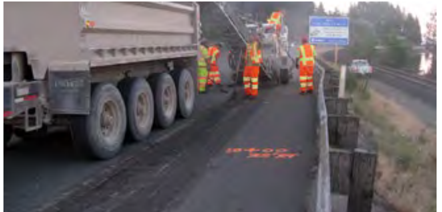
Low-cost safety strategy: rumblestrips
