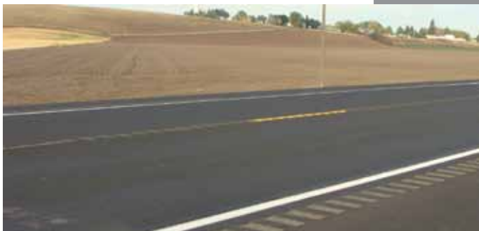
Combination rumble strips help reduce the potential for cross over crashes related to driver inattention, falling asleep, distracted driving, etc.
