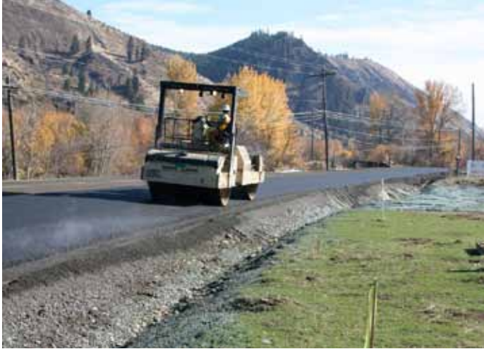
SR 410 Nile Valley Landslide in November 2009 resulted in an emergency route. Preliminary construction of a permanent fix has begun.
