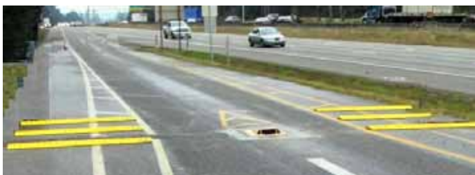
Speed bumps and pavement markings guide trucks over the AIRS thermal imaging camera embedded in the weigh station approach lane.
