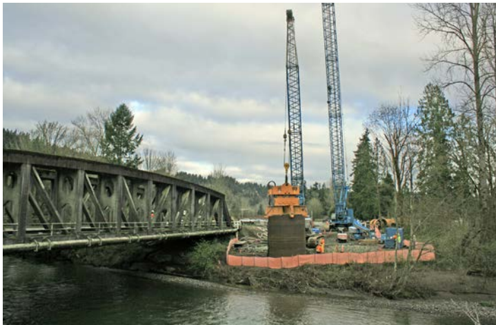
Contractor crews working for WSDOT in the process of rebuilding a new bridge on State Route 162 across the Puyallup River Bridge in Pierce County.
