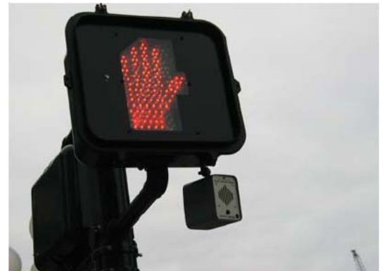
Exhibit III-1.14 – An Audible and Visible Pedestrian Signal (Location: Bellevue, WA)
