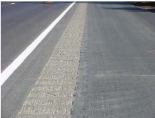
Exhibit V-3.8 – Shoulder Rumble Strip (Location: I-5, WA)
