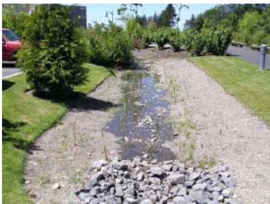
Exhibit V-13.5 – Pierce County Public Works Building Stormwater Treatment Facility (Location: University Place, WA)
