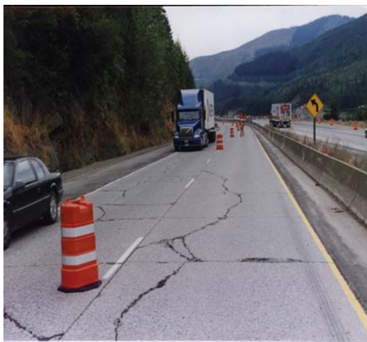
Exhibit A-10.4 – Deteriorating Pavement on Existing Route
