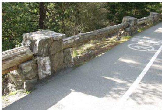
Exhibit IV-4.4 – Historic Civilian Conservation Corps Rail (does not meet current day design requirements) (Location: Deception Pass, WA)
