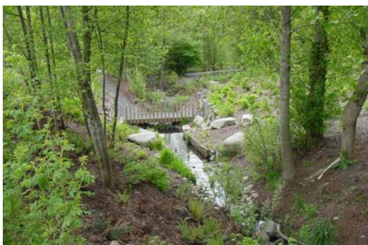
Exhibit IV-2.3 – Stormwater Facility (Location: Indian Creek, Olympia, WA)
