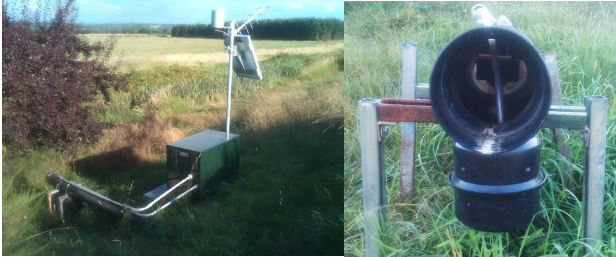
Figure 12 Everett MVFS DCP with views of sampling and gaging pipe equipment.
