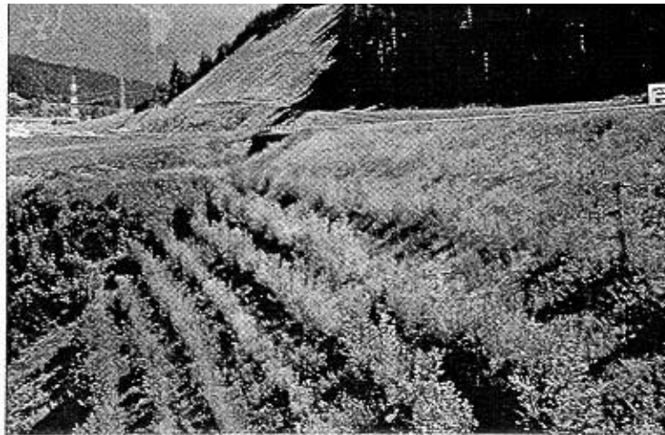
Figure 7. Brushlayer embankment fill stabilization after two years showing both grass and brush establishment. Brenner Pass highway, Austria.
