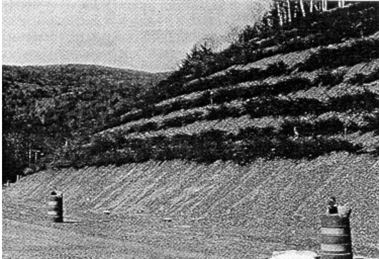
Figure 4. Brushlayer buttress fill immediately after construction . Winter 1990. Greenfield Rd., nr. Route 112, Colrain, Mass.
