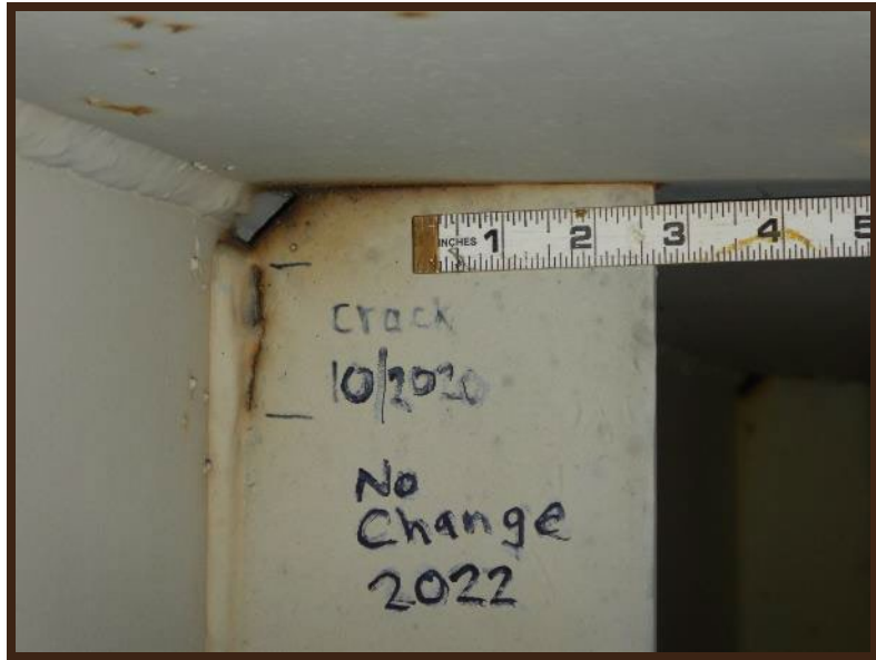
Crack in the top of a longitudinal stiffener
