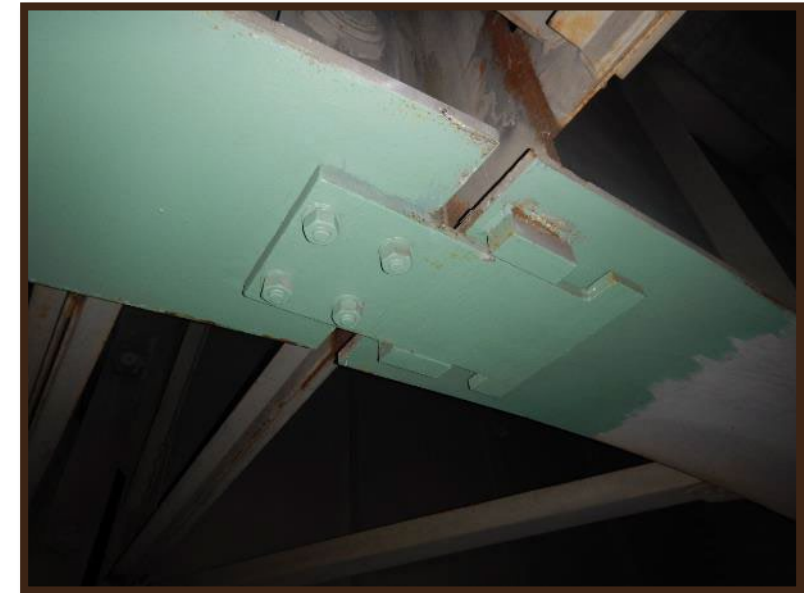
Weld Replaced with Bolts
