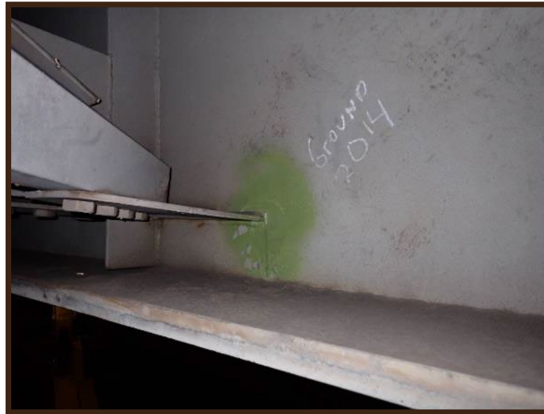
Ground Out Crack
