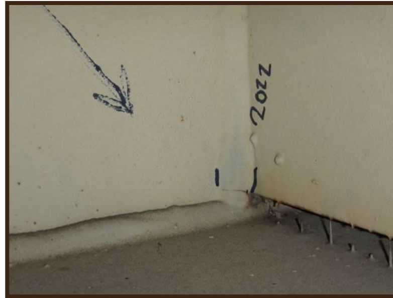
Crack in the toe of a longitudinal stiffener
