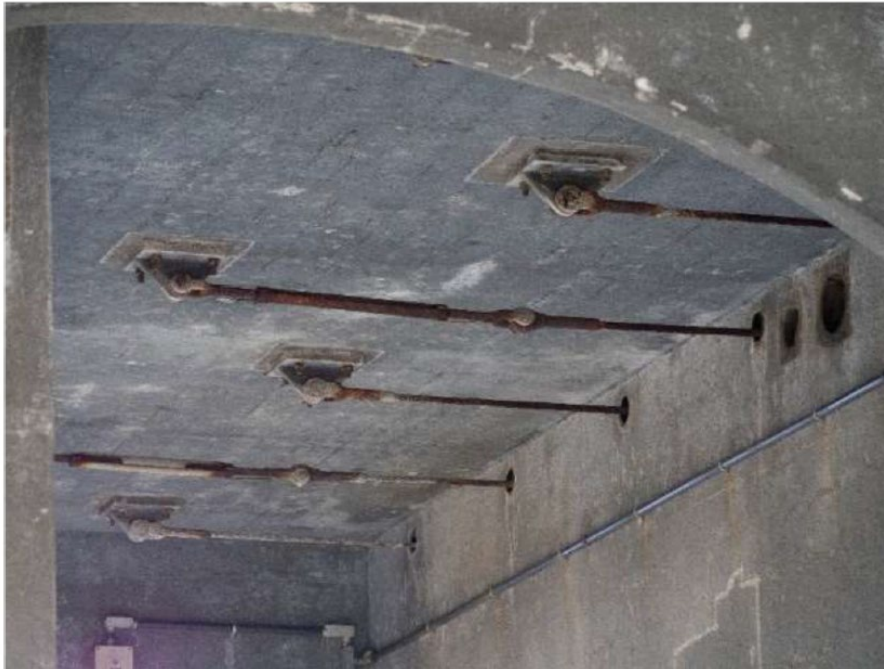
Figure 1: Example of corroded seismic restraint cables.
