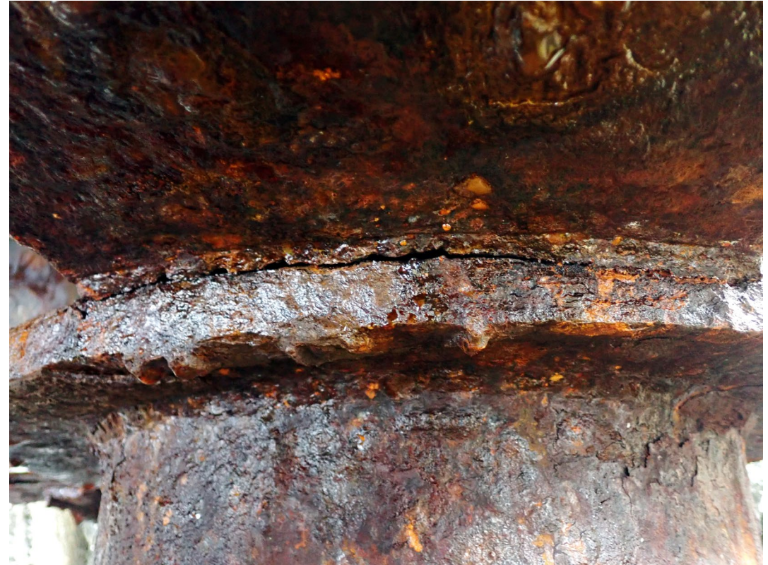
Crack at the Girder to Base Plate Weld
