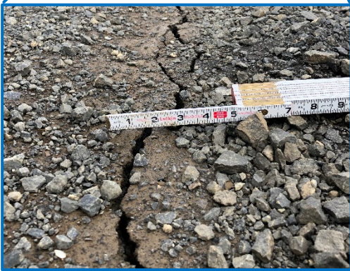
Soil Cracking in Breakwater
