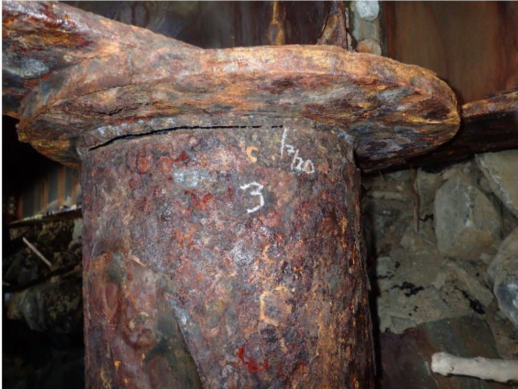
Crack at the Pile Weld
