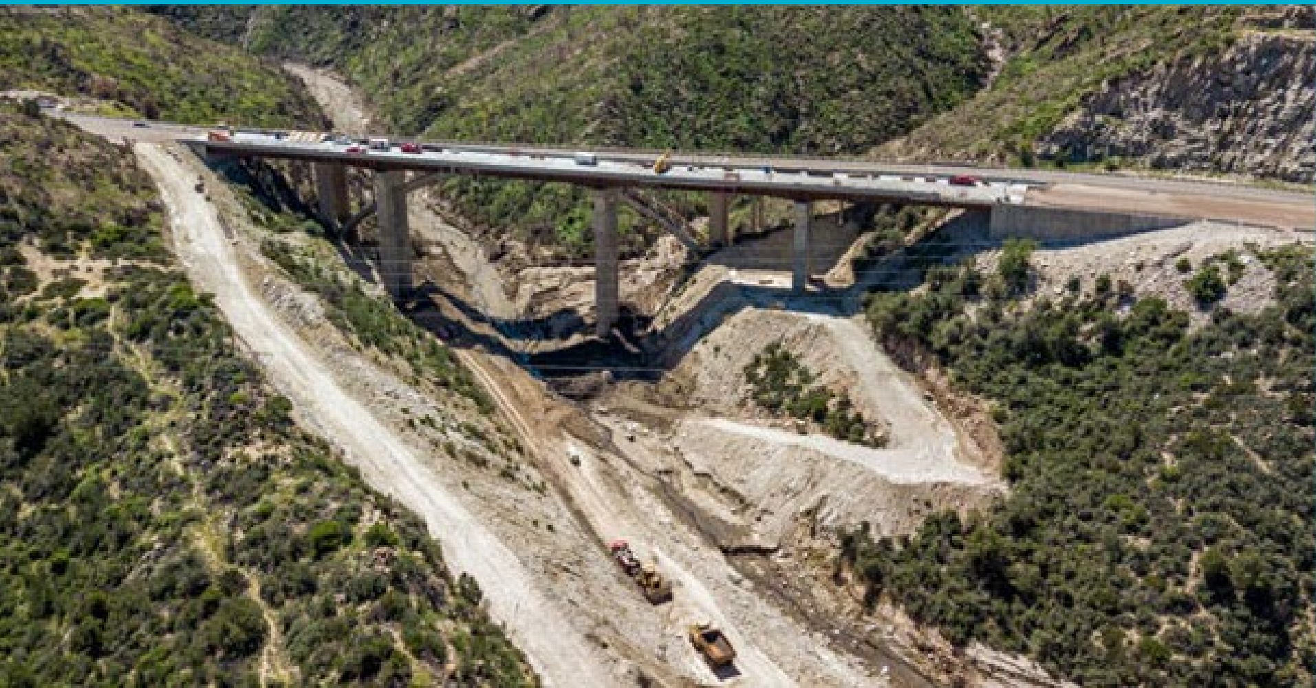
Pinto Creek Bridge blowout of construction site. Pumphouse wash had a larger watershed and faster velocities
