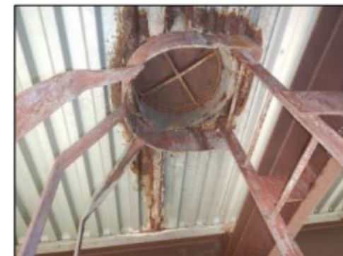
Corrosion on SIP Forms
