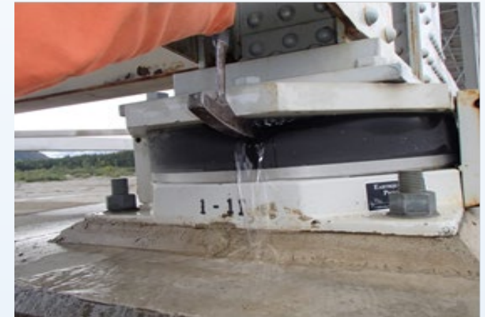
Water contamination in FPS bearing Source: Alaska DOT&PF
