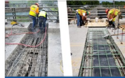
Replacement of an expansion joint with a UHPC link slab. Source: New York State Department of Transportation
