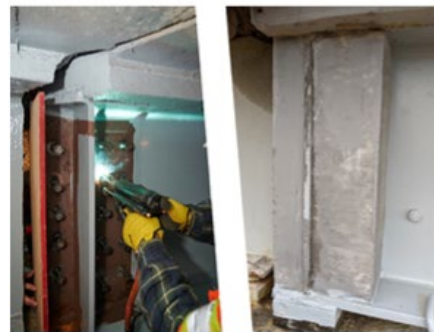
Repair of a deteriorated steel bridge beam end using UHPC. Source: University of Connecticut
