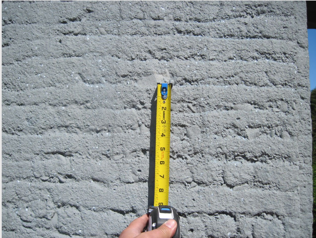
Damage from sand blasting
