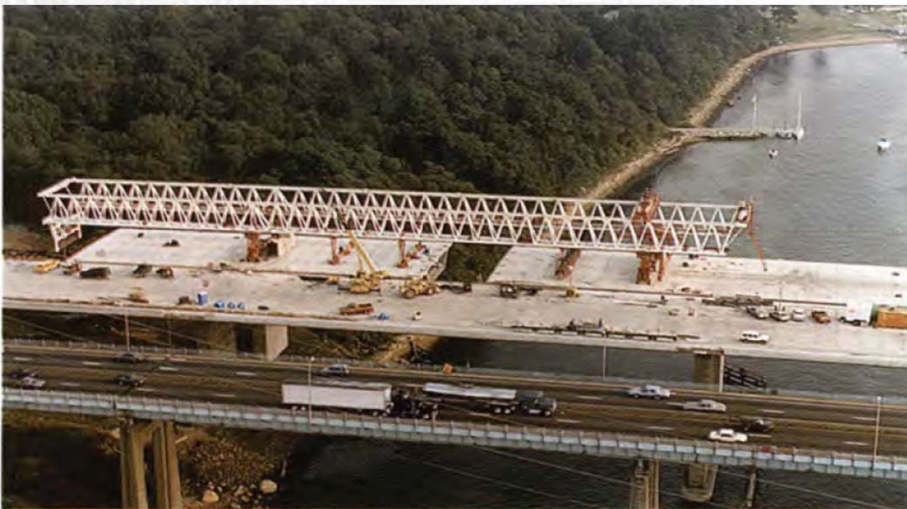
Fig. 29. Final segments being placed in last span of new, parallel segmental bridges; existing bridge is in foreground. From PCI Journal
