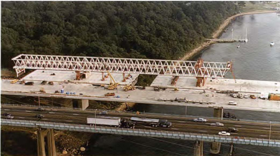
Fig. 29. Final segments being placed in last span of new, parallel segmental bridges; existing bridge is in foreground. From PCI Journal
