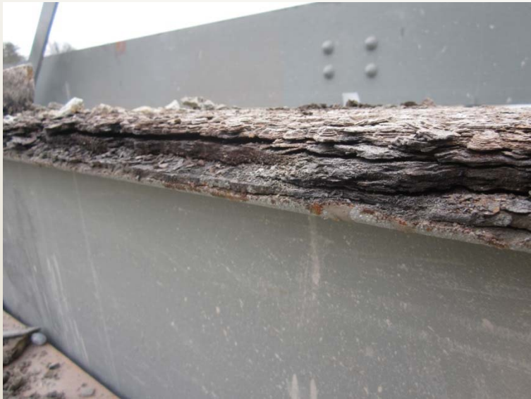
Before Cleaning Stringer
