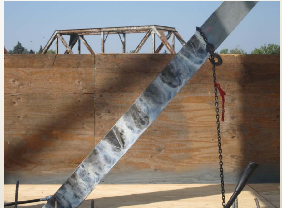
After Heat Straightening
