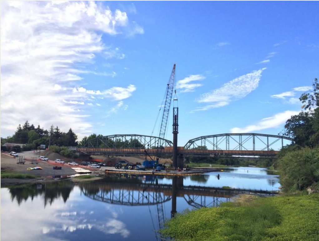
Pile Driven In Close Proximity to Existing Bridge to Limit Span of Bent
