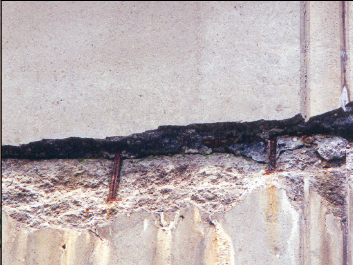
Failed Concrete Next to Joint Due to Corrosion
