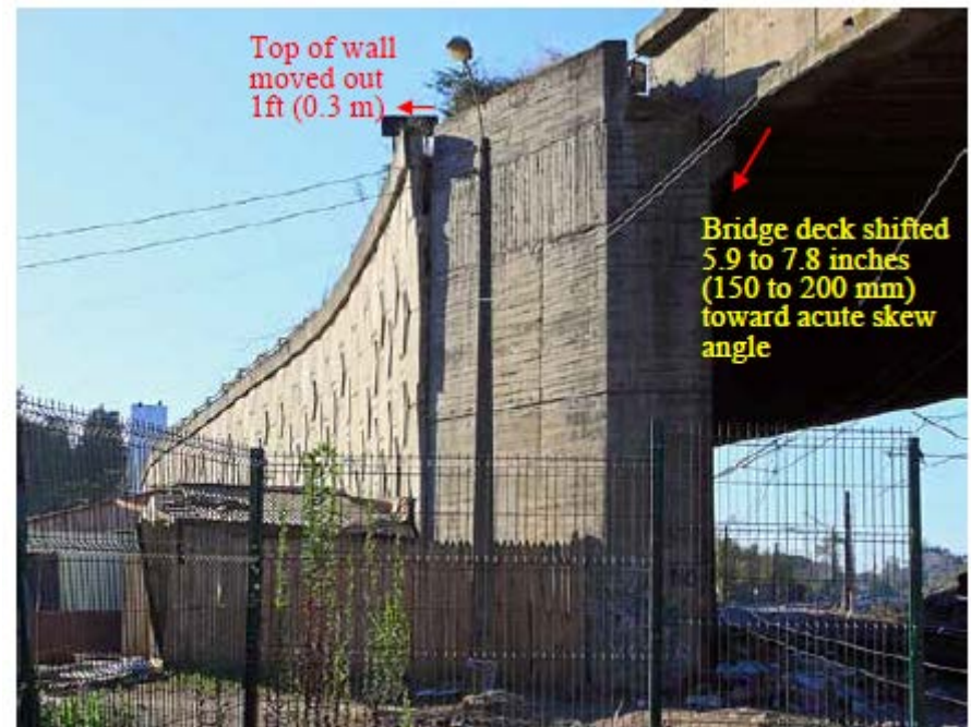
Figure 268. Photo. Wall corner tilting outward at wall site 28B.
