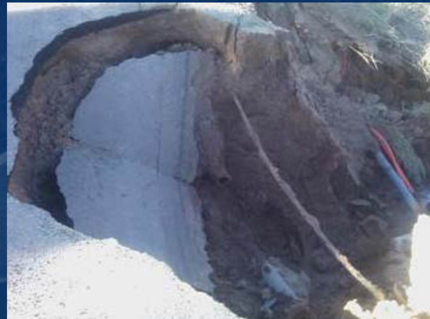
Close-up of failed area of Drew Road, April 2010
