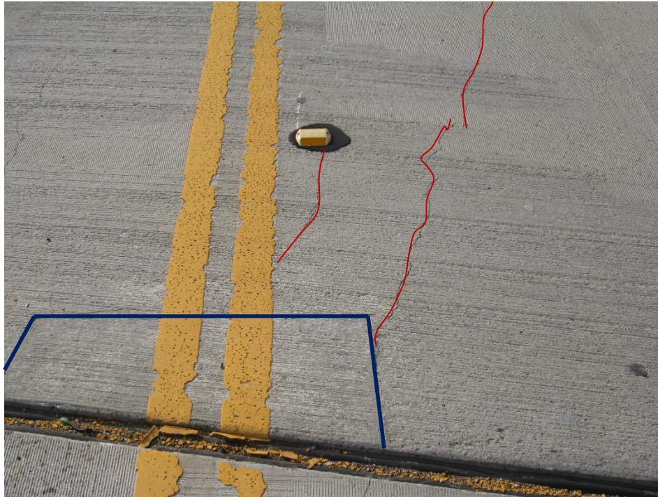
Cracks developed out of the block-out corner
