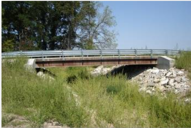
Audrain County, MO Bridge 411 Built 2012 Steel 4 Girders 47.5 ft. Span 24 ft. Roadway Width 2 ft. Structural Depth No Skew
