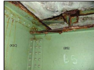
PIER 5 (B5) TOP FLANGE
