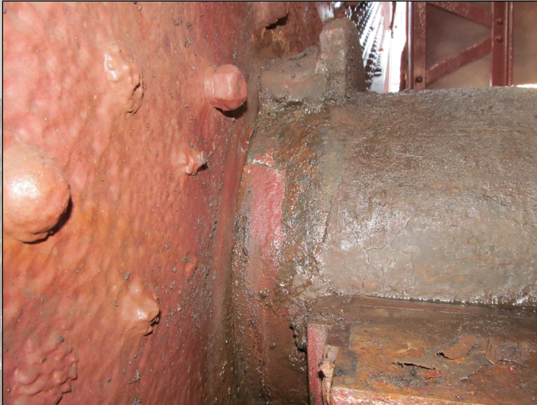
Outboard bearing – fractured steel collar
