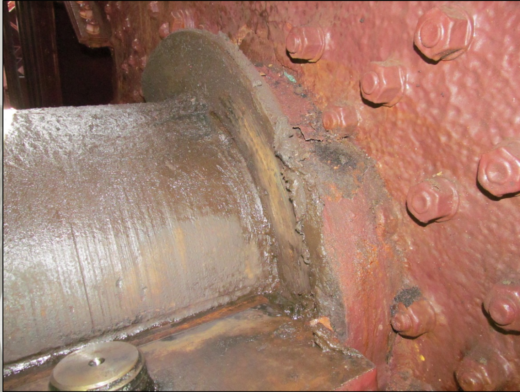
Outboard trunnion journal – grease groove nearly worn away at inboard end
