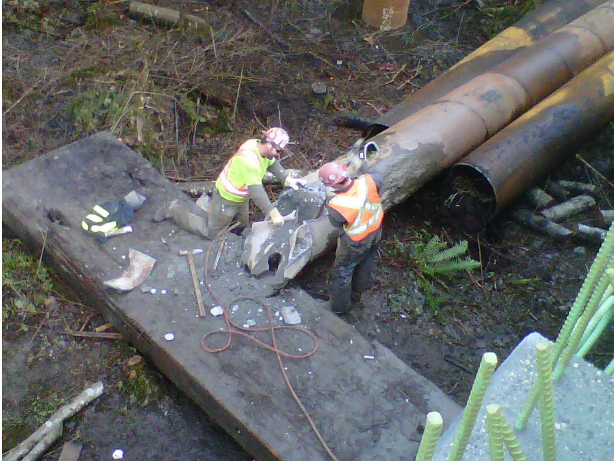
Pile tip damage
