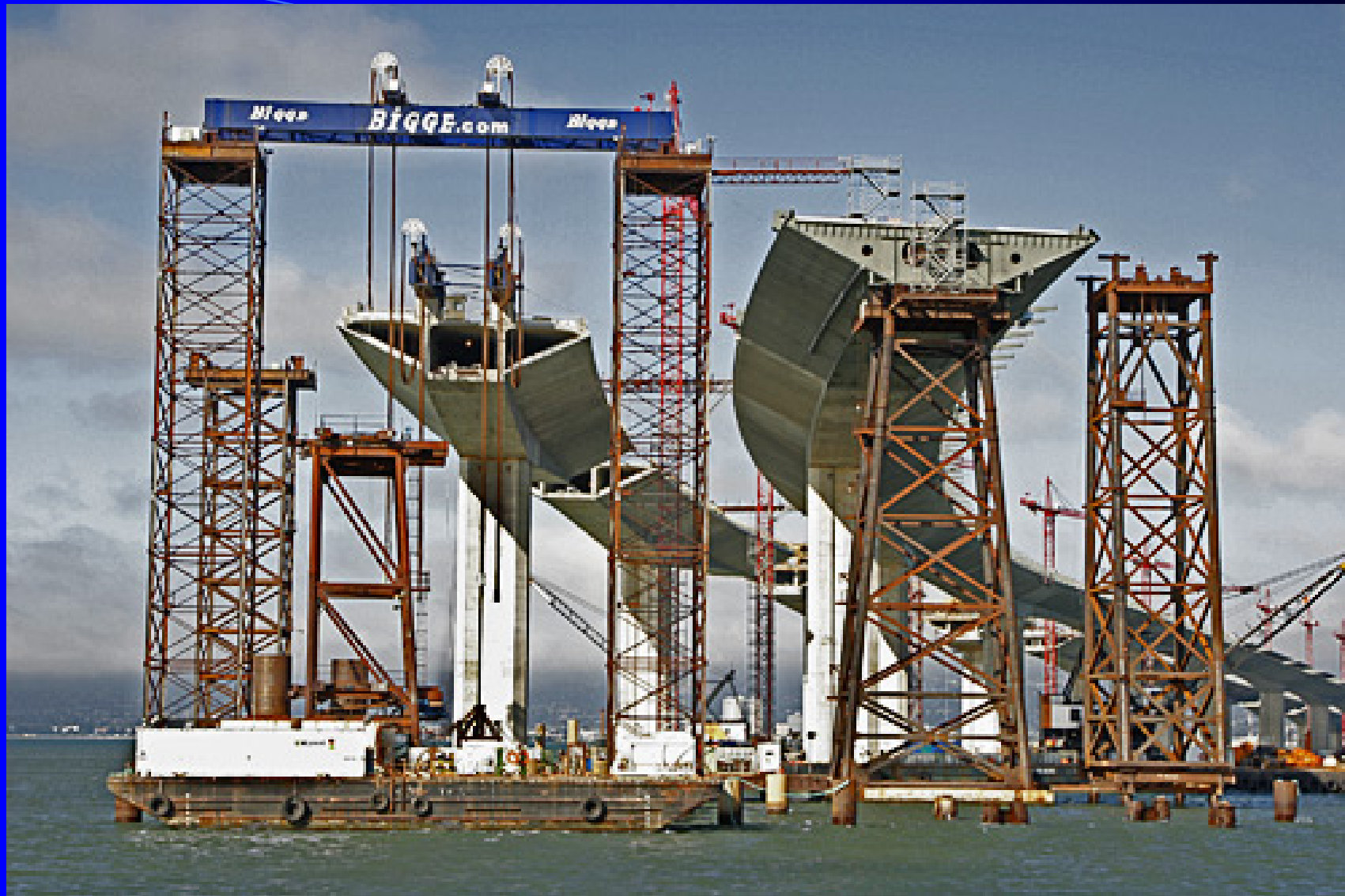
Lift of Skyway Orthotropic Spans – Fabricated by Universal Structures Inc and Oregon Steel
